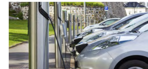
Electric Vehicle Charging Point
